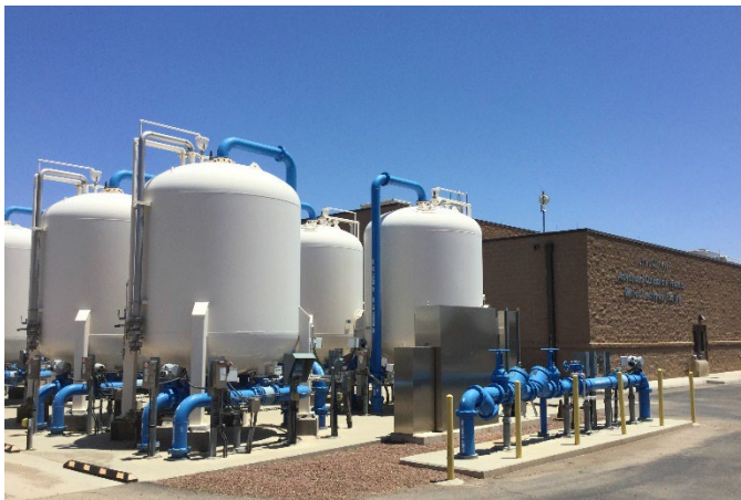
Caption: Tucson Airport Remediation Project facility.
