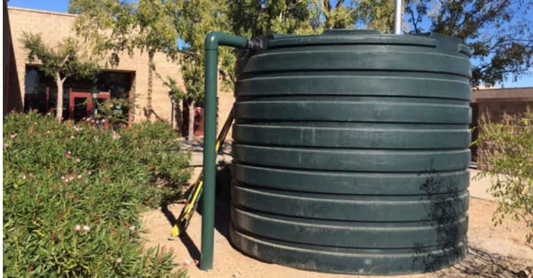
Caption: Rainwater Harvesting Cistern at the Ward 5 Council Office.
