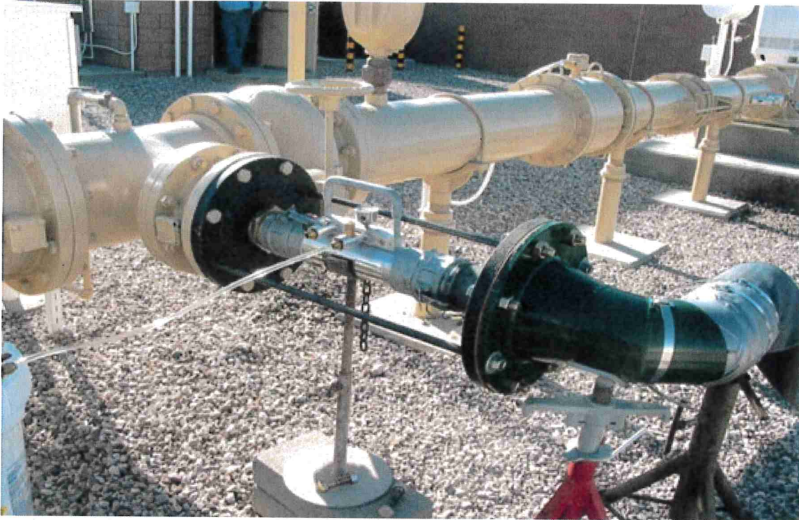
Romac Venturi Device to feed ascorbic acid for de-chlorination. (0-200 ppm)
