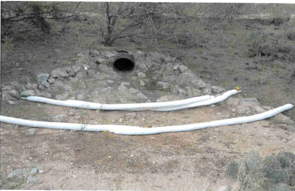
Reservoir out fall with absorbent socks. Installed to perform similar to straw wattles to capture any oil sheen. Image from Andy Vanover, Tucson Water ( January 2008)
