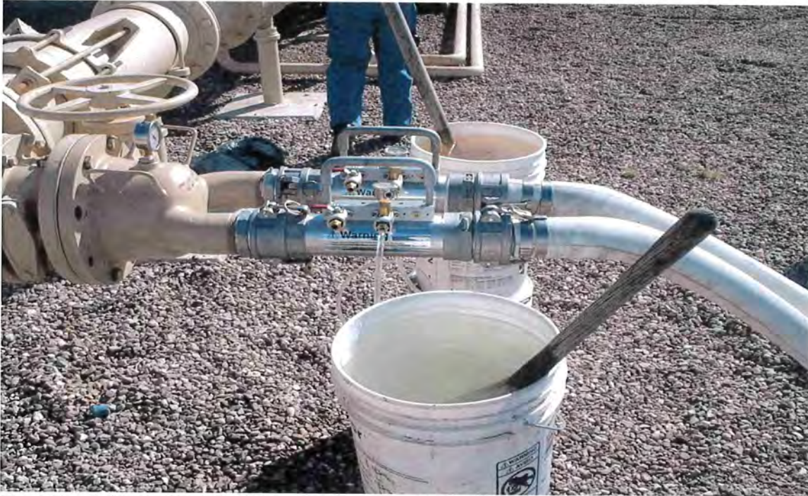
Two Venturi Manifold for flows greater than 1800 GPM – CA-009A De Chlorination Image from Andrew Vanover , Tucson Water.
