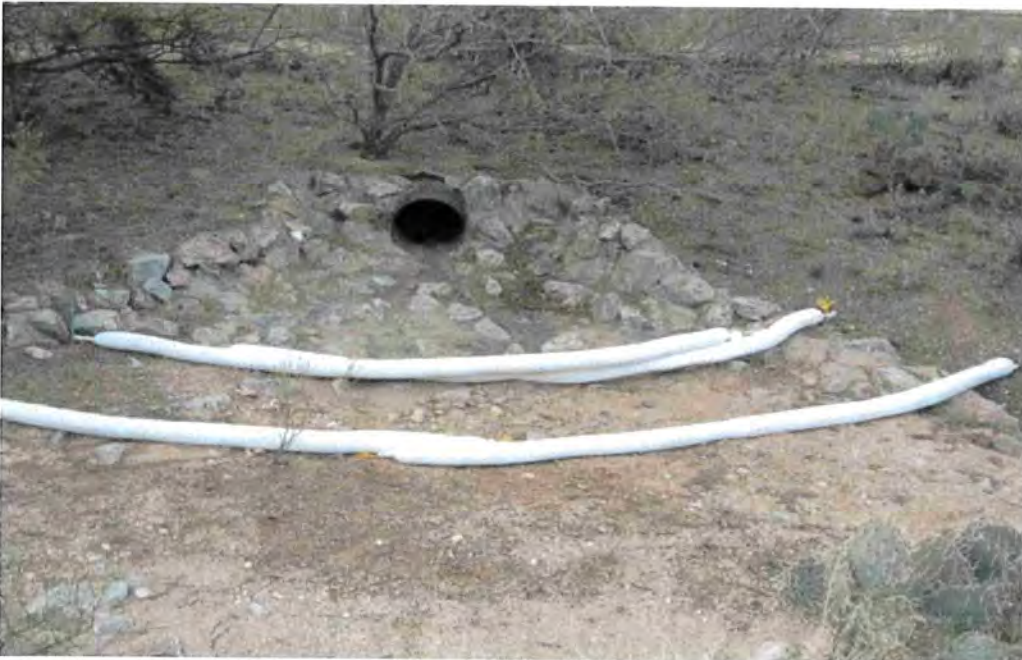
Reservoir out fall with absorbent socks. Installed to perform similar to straw wattles to capture any oil sheen. Image from Andy Vanover, Tucson Water ( January 2008)
