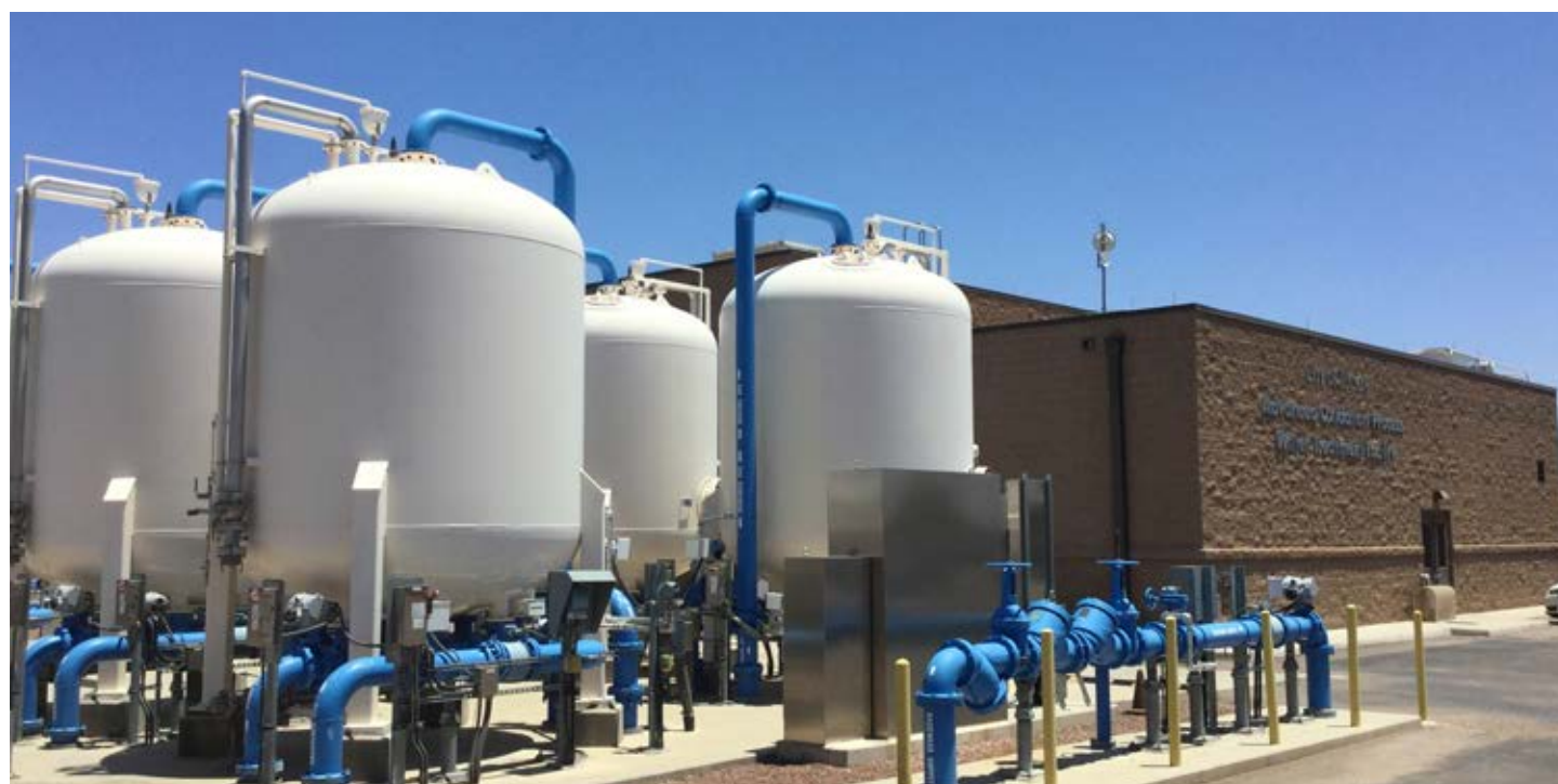
TARP ADVANCED OXIDATION PROCESS (AOP) FACILITY
