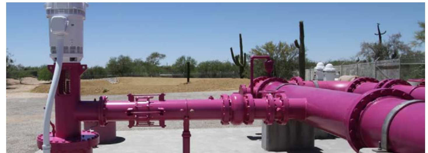
“PURPLE PIPES” IN THE RECLAIMED WATER SYSTEM
