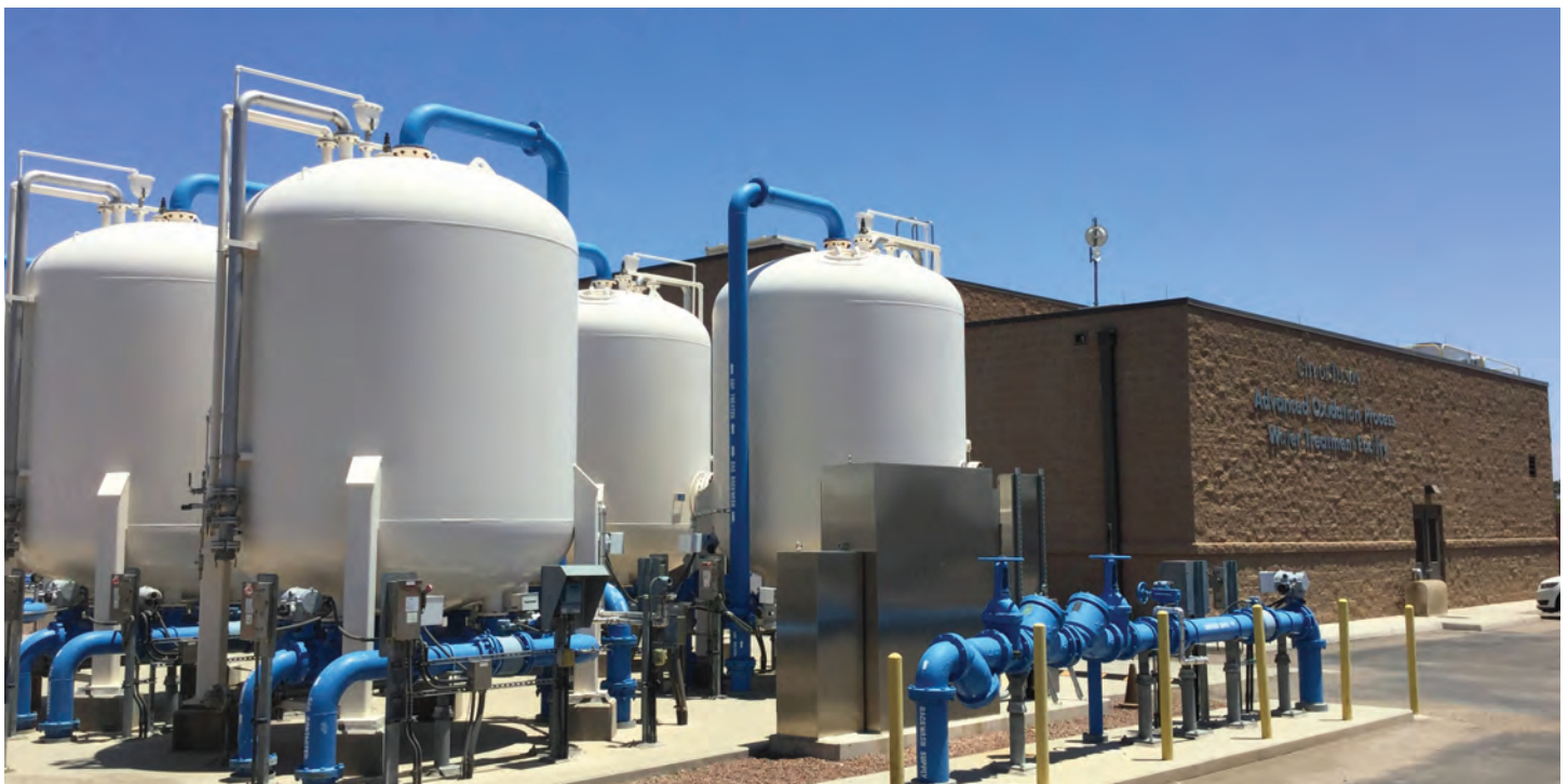
TARP ADVANCED OXIDATION PROCESS (AOP) FACILITY
