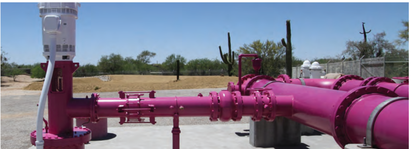
"PURPLE PIPES" IN THE RECLAIMED WATER SYSTEM
