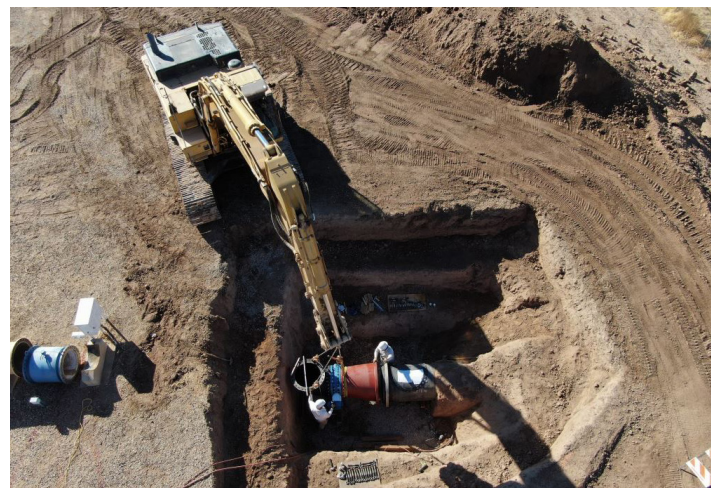
CAVSARP valve installation, Water Bank of Tucson
