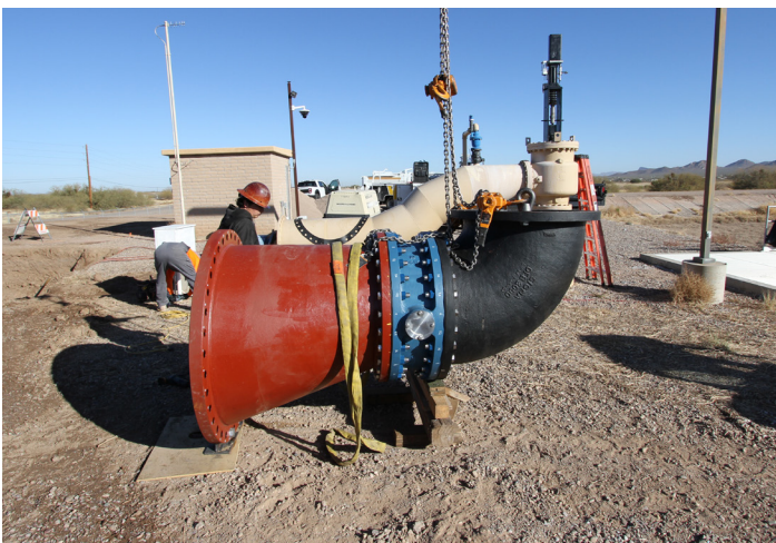
CAVSARP replacement valve
