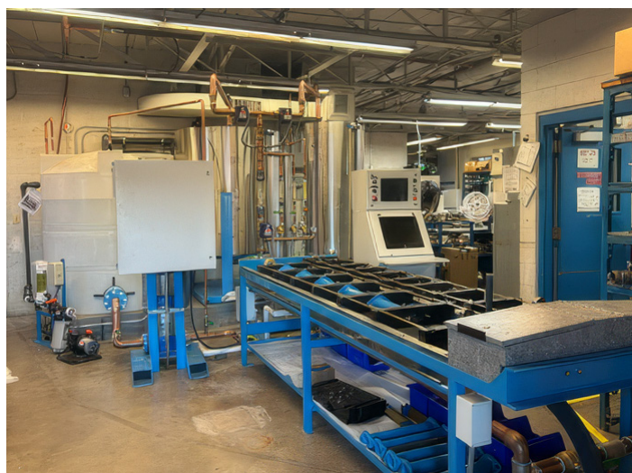
New meter bench improves the ability to test multiple meters including ultrasonic.
