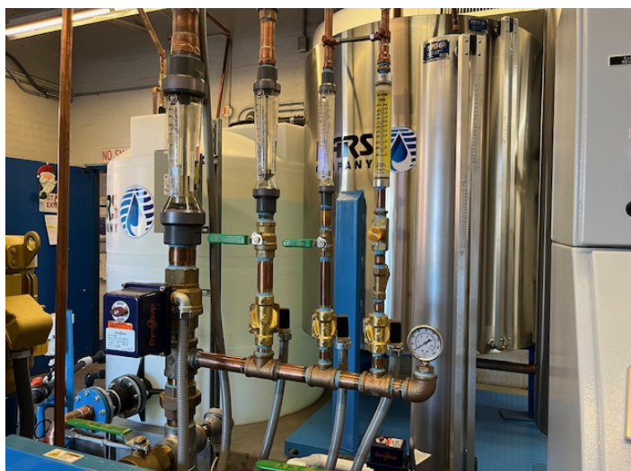
Meter bench test tanks save water by storing recirculated water during testing.
