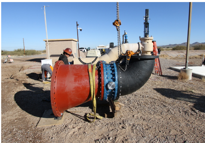
CAVSARP replacement valve
