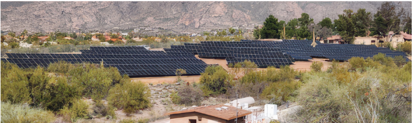
Tucson Water Solar Project
